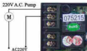
Figure 3-7 Wiring of Booster Pump on Inlet
